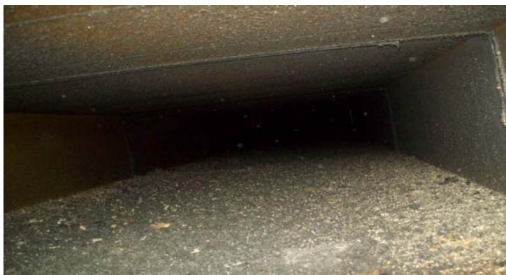
Internal duct surfaces of general ventilation system showing accumulation of dust and debris
