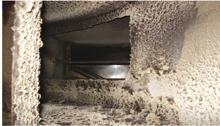
Internal ducting surfaces of grease extract system showing uncleaned potentially flammable grease deposits
