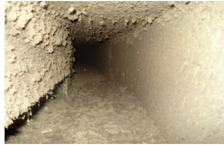
Internal surfaces of air conditioning duct showing accumulation of dust and debris
